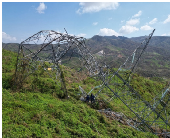
Photo 11: Collapsed transmission tower after Hurricane Otis, Mexico, with surveying personnel conducting the corresponding technical assessment in the field, 2024. Photograph courtesy of Federal Electricity Commission of Mexico.
