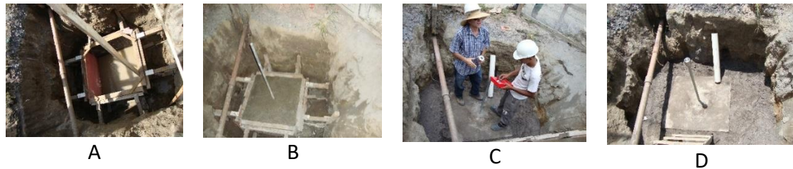
Figure 3: Level References of the LITPEG construction. A. Construction of RN LITPEG01; B. Concrete of the base and fixation of metal rod; C. Fixation of BM; D. RN LITPEG01 and support of the invar leveling rod. Data:23/09/2015.
