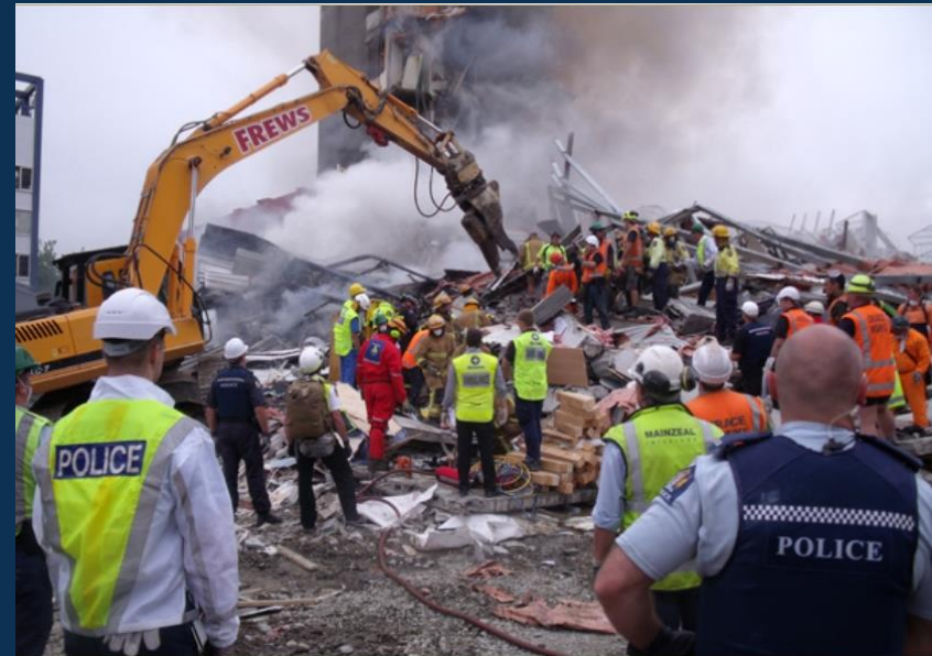
Buildings & facards collapsed
