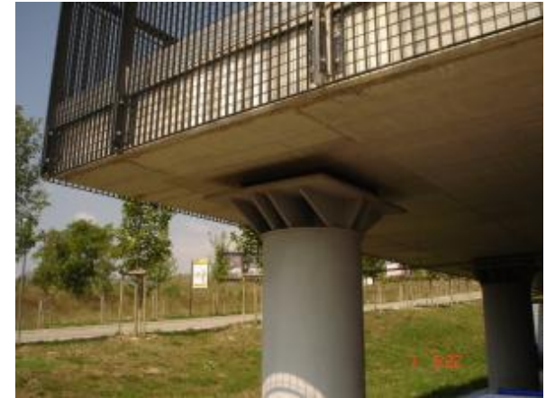
Seismic isolation in Bazzano, new settlement built around L'Aquila, 2012.
