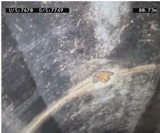
JF-L due to minor concrete damage at joint. IRTS&G requires repair to DN1800 pipe.
