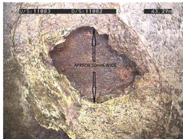
PH-L – historic repair with steel plate sealing hole prior to backfill.
