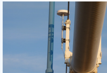
AT503 Antenna Attached to Main Cable on Severn Crossing Suspension Bridge
