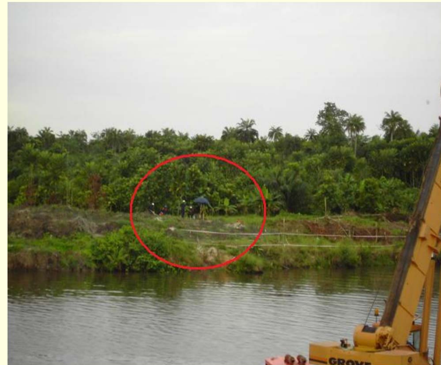
Survey crew on site during EPS site layout setting out and preparation.
