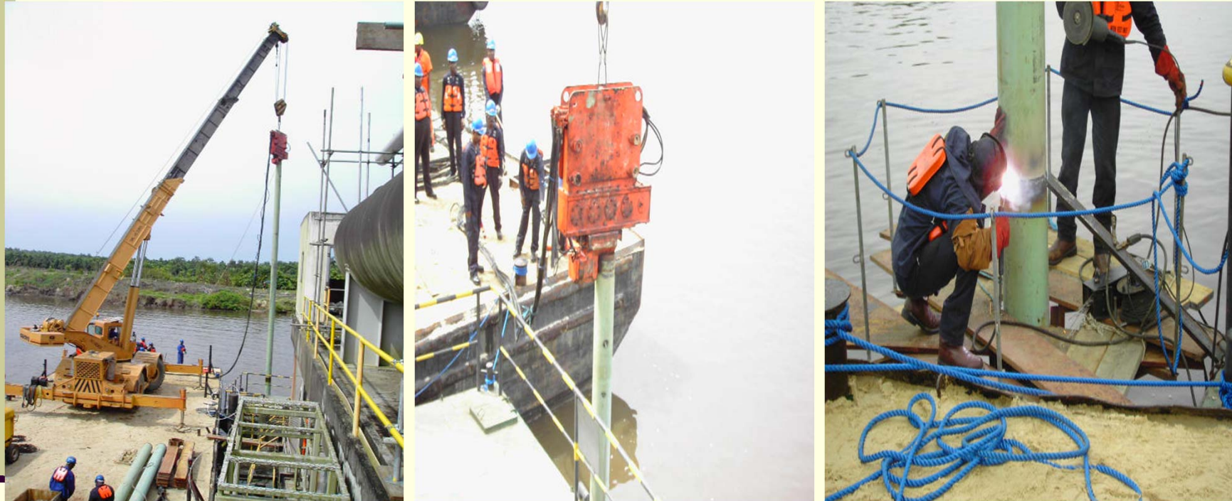
Installation of 16nos 12" double length Piles using vibro pile hamper and Welding work at the EPS barge location
