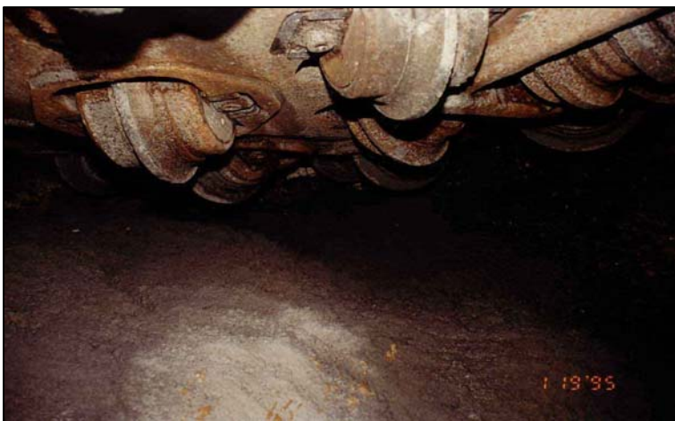
Fig. 5: Close-up of the rotary bit. The borehole diameter is 5 m. Photo E. Meier.
