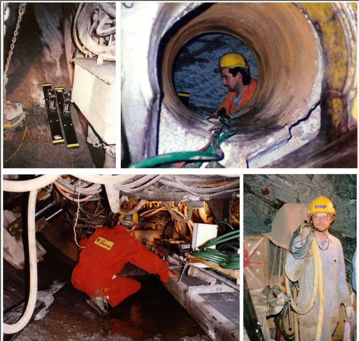
Fig. 6: GPR 100 MHz antennas (top left), Manhole with fibre optics (top right), engineers passing GPR equipment through a manhole (bottom left) and carrying protection tubes for the vulnerable fibre optics (bottom right). Photos: E Meier, U. Sambeth.
