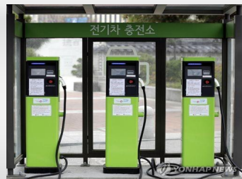
* electric vehicle charging station
