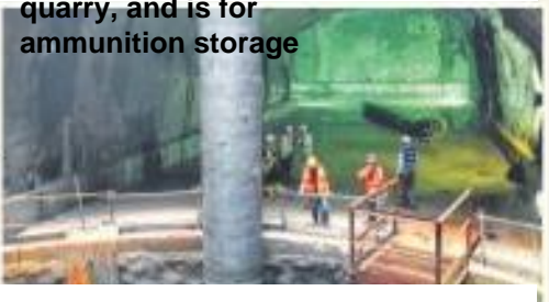
Jurong Rock Cavern It is being built 130m below Banyan Basin on Jurong Island to store crude oil and other petroleum products
