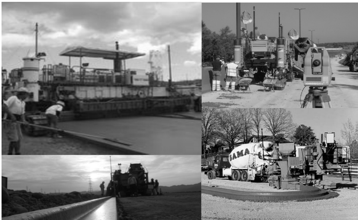
Figure 7: Leica LMG S System, Slipform Paver, Barrier Paver, Curb and Gutter Application
