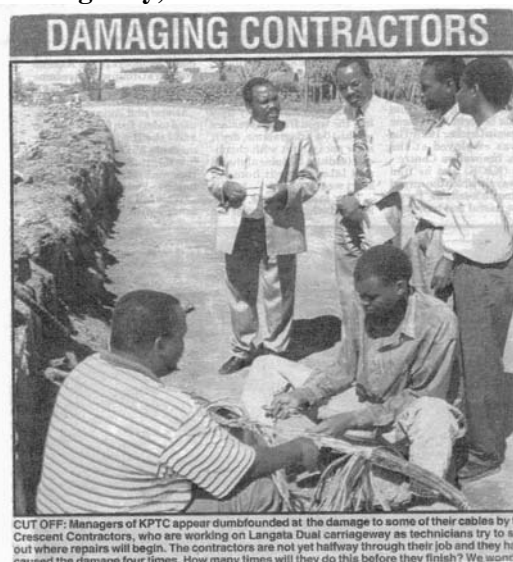
Photograph 1: KPTC Cables damaged during the construction of the Langata Dual Carriageway, Nairobi.
