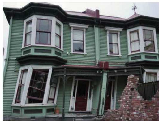
▲ The 2010 and 2011 earthquakes caused major structural damage to Christchurch.
